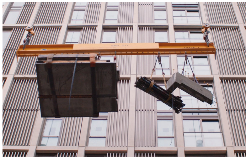
FIGURE 11: Gantry crane with twin 15t hoists to lift full precast sections to working face
